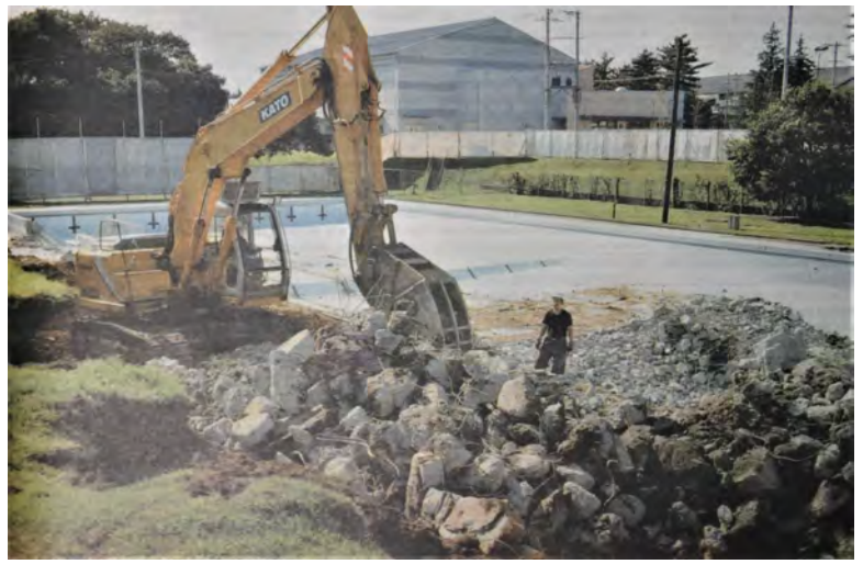
Demolition of the Camp Zama outdoor swimming pool facility continues Sept. 19, 2002, as work crews tear up concrete and plumbing. This pool was no longer needed when the Yano Fitness Center opened with its year-round indoor swimming pool.
