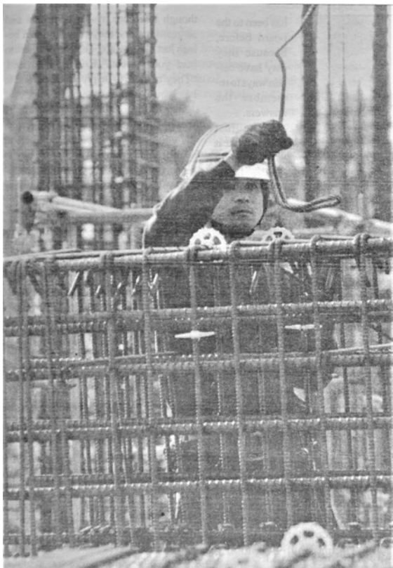
(Left) In January 2000, Ryuji Moromi prepares to hook up a rebar frame for lifting into place. The frame will go into supporting the walls of the Yano Fitness Center.
