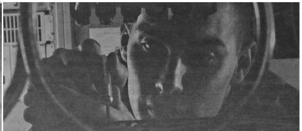
Air Force Airman 1st Class Kevin Becker, systems control journeyman, installs cross-connects for a new technical control data circuit in November 2004. Becker is assigned to Location C, 374th Communications Squadron, at Camp Zama.
