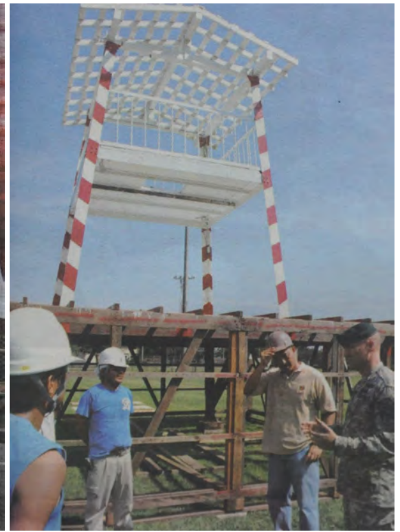
Colonel Robert M. Waltemeyer, U.S. Army Garrison Japan commander, talks with Department of Public Works employees during Bon Odori tower construction July 24, 2008.
