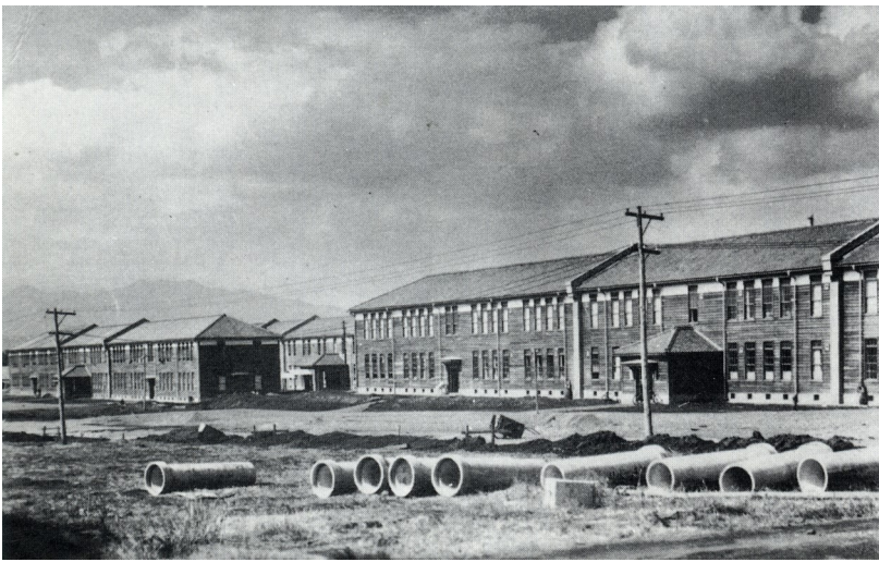
Sewer pipes waiting to be laid below ground line an area in front of some nearly completed buildings.
